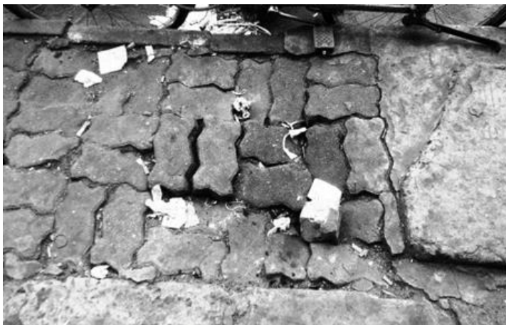
Figure 3: Poor condition of pavement (source: Barua et al., 2007)
